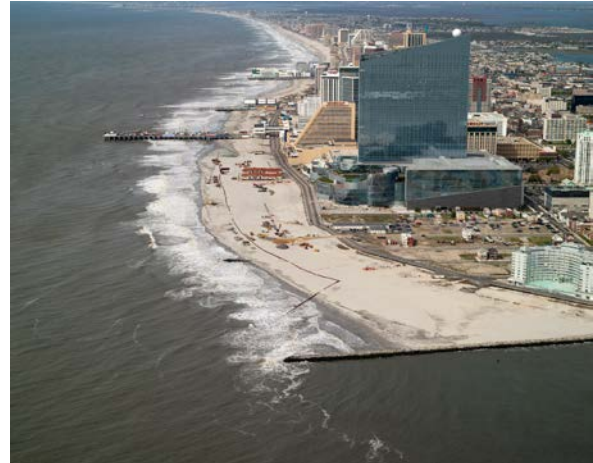
The U.S. Army Corps of Engineers Philadelphia District pumps sand onto the northern end of Atlantic City in 2012 as part of the first full scale renourishment of the project.
