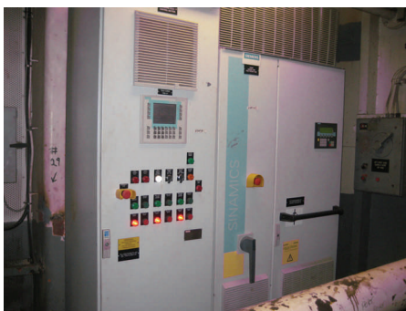
New Dragarm Winch Motor VFD
