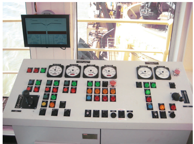
Dragarm and Pump Control Console (After)
