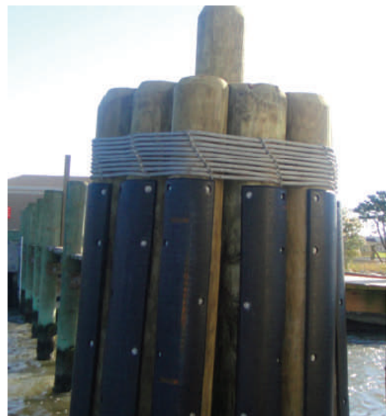
19-pile timber dolphin faced with UHMW Polyethylene fendering in Ocean City, MD.
