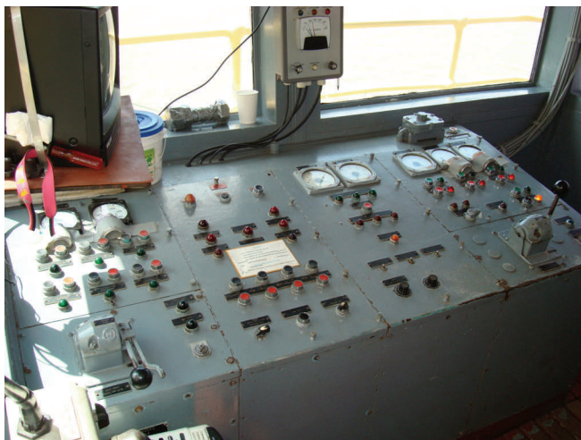
Dragarm and Pump Control Console (Before)
