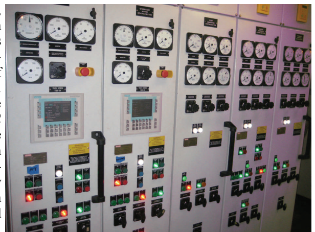
New Dredge Pump Switchboard
