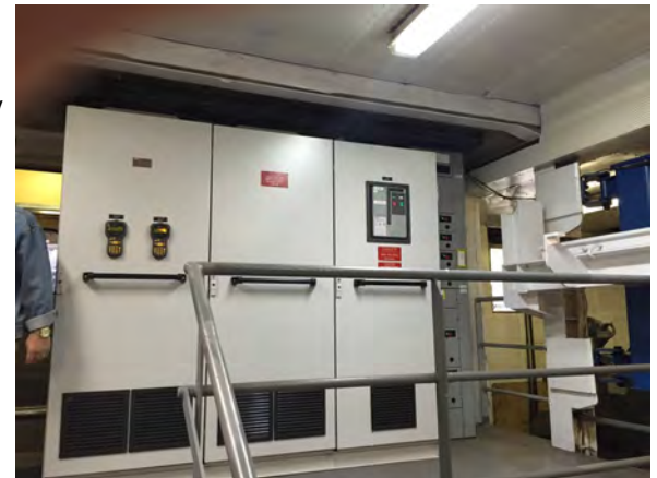
Dredge HURLEY VFDs
