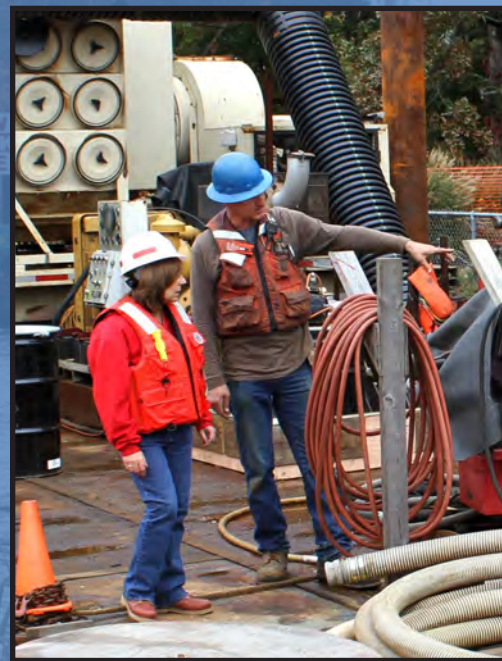
Rudy Sorrells, an inspector for Abhe & Svoboda, speaks with Monica Chasten, a project manager for the U.S. Army Corps of Engineers Philadelphia District. Sorrells explains the operation of a desalination station used to produce freshwater for an ultra-high pressure wash of the steel bulkhead along the Point Pleasant Canal.
