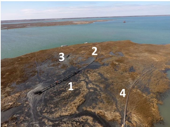
Northern portion of Sturgeon Island showing (1) elevated pipe distribution system; (2) Y-valve flow separator; (3) spreader system; and (4) elevation-controlling containment pipe.
