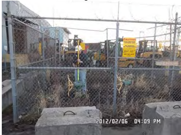
Transco Gas (Williams)-west-NJ-looking north
