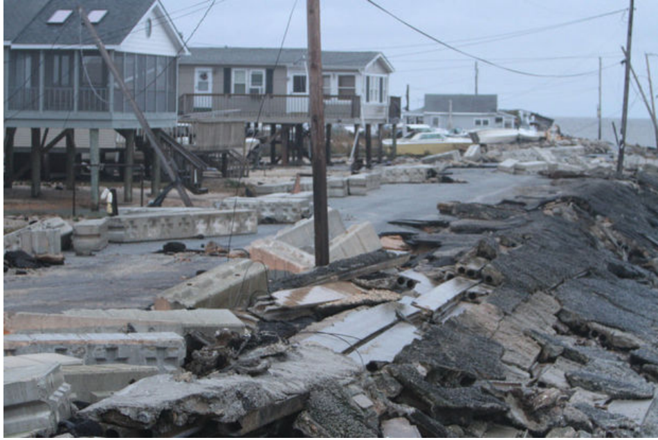
Photo 7: Damage following Hurricane Sandy in Gandys Beach
