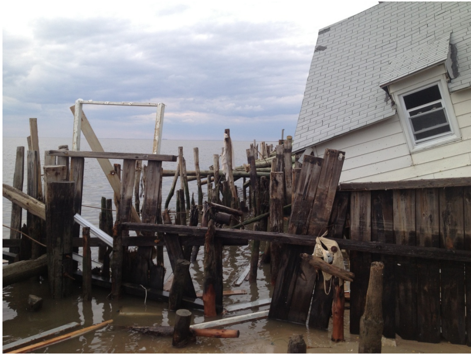
Photo 4: Damage following Hurricane Sandy in Fortescue
