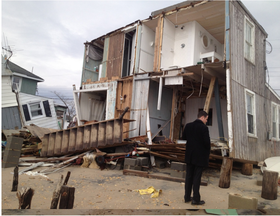
Photo 3: Damage following Hurricane Sandy in Fortescue
