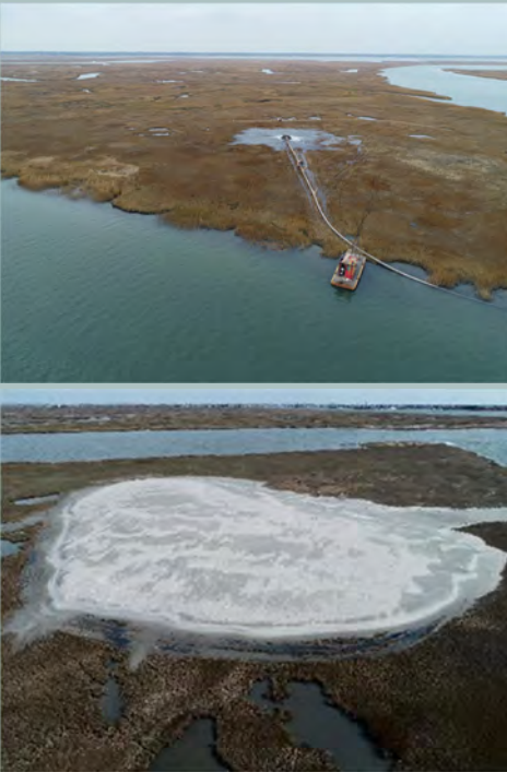
Habitat Creation at Great Flats, near Stone Harbor NJ conducted as part of the NJIWW dredging and beneficial use placement project in December 2018 and again in February 2021. Barnegat Bay Dredging from Harvey Cedars, NJ was contractor for this and several innovative placement projects done through collaboration with the State of NJ.
