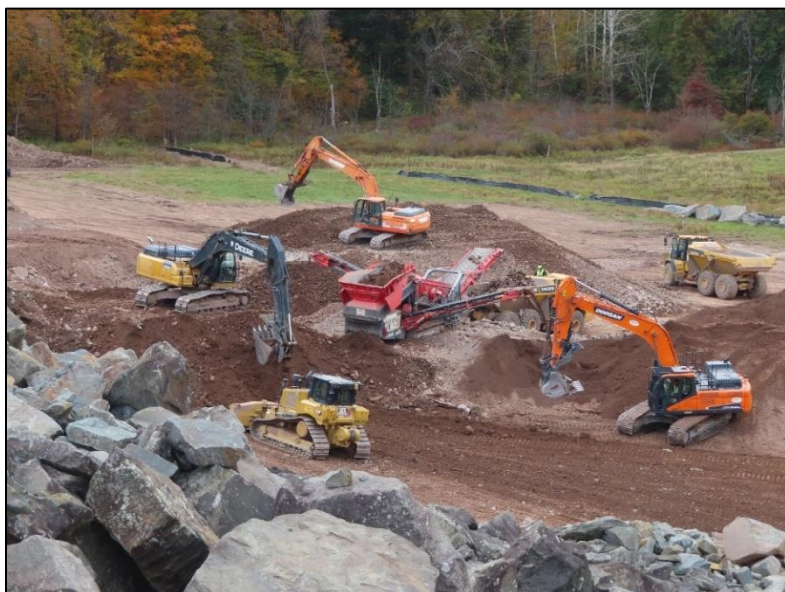
JADWIN DAM: The U.S. Army Corps of Engineers and its contractor constructed a Dam Safety Modification project at Jadwin Dam in Wayne County, PA. Work involved the installation of a geosynthetic liner system on part of the upstream slope and crest of the dam.
