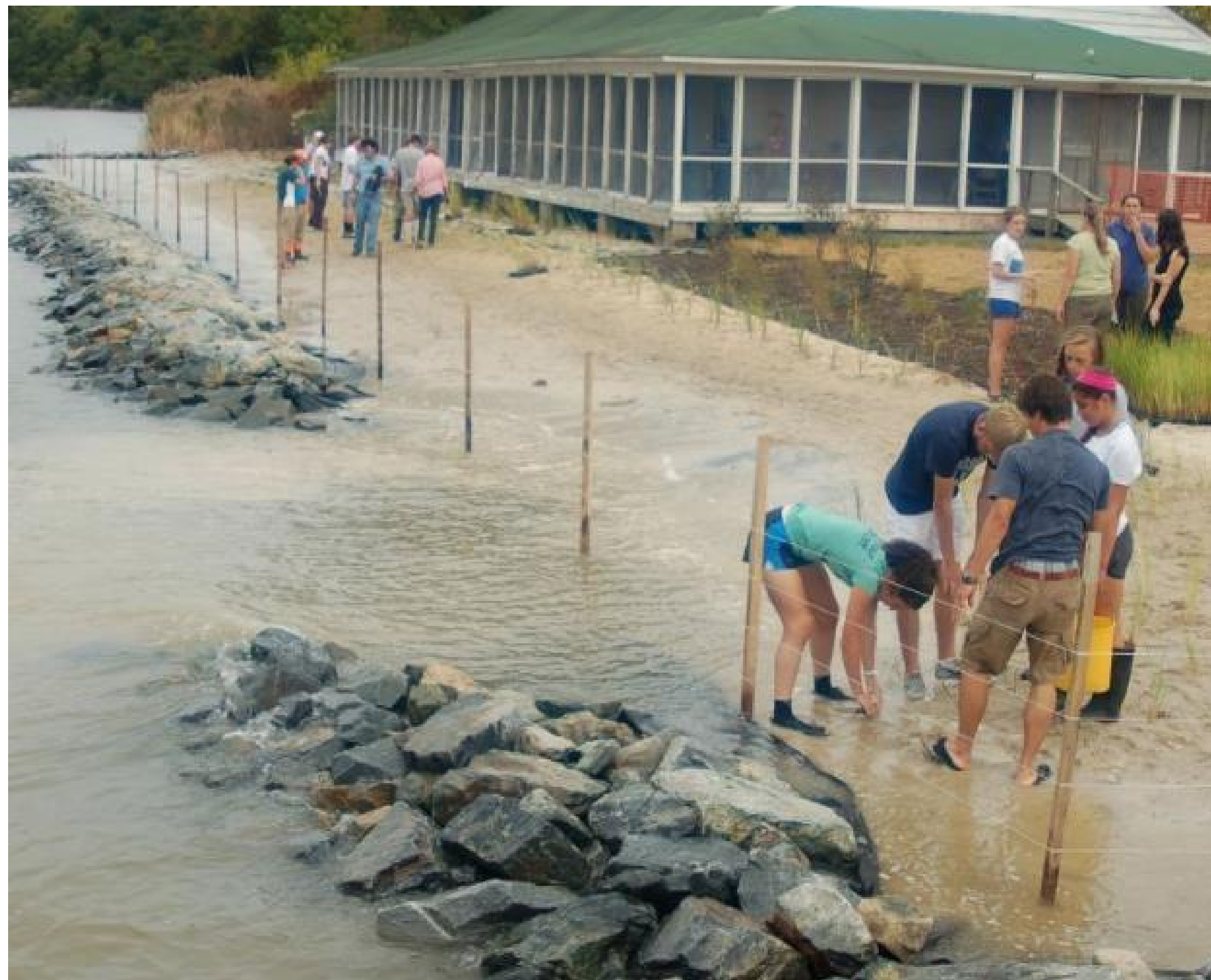
Construction of living shoreline in Camp Pecometh, MD. Image source: Jack Shaum, MyEasternShoreMD
