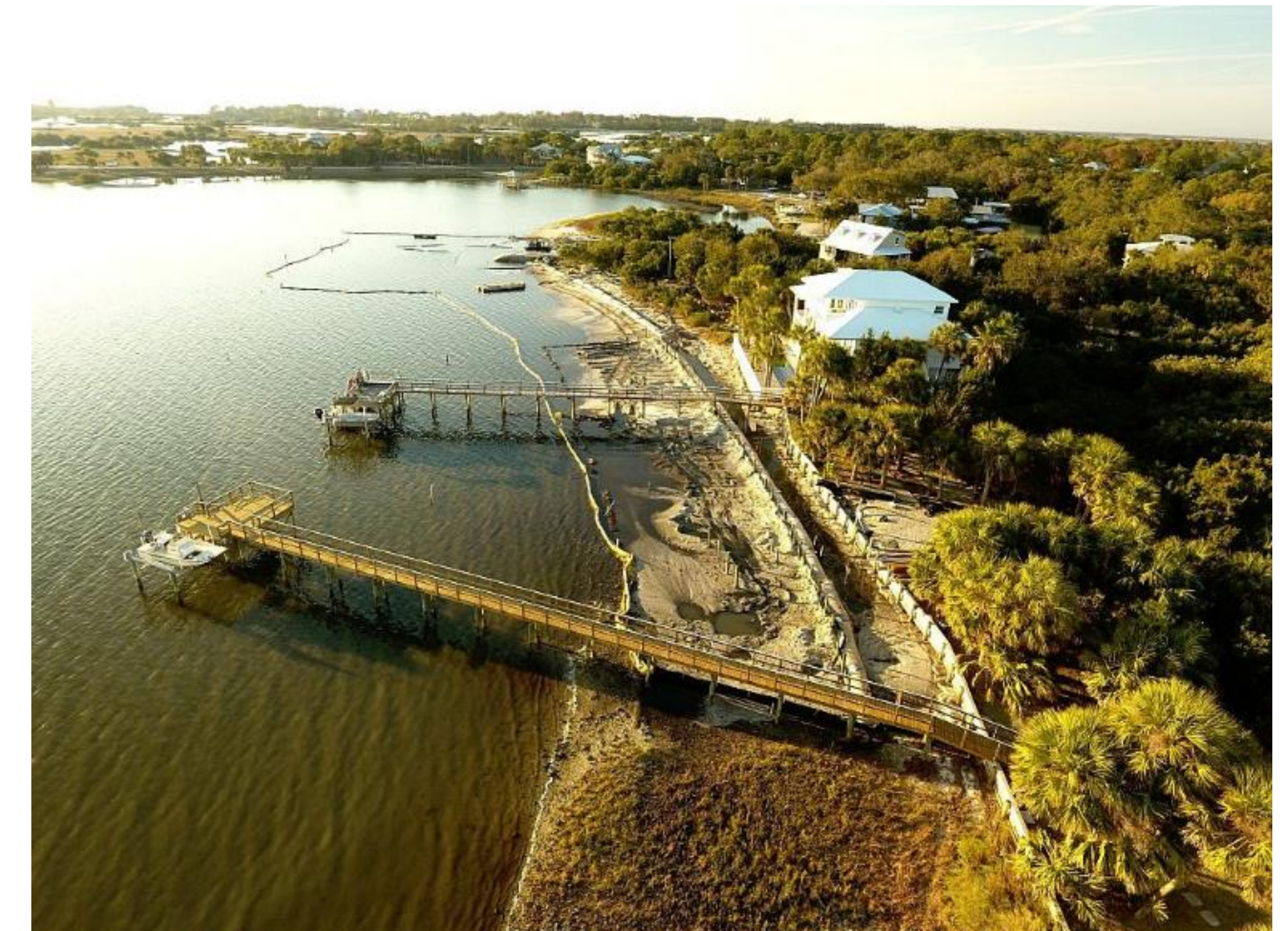
Construction of living shoreline in Cedar Key, FL. Image source: Dr. Mark Clark; University of Florida, Nature Coast Biological Station
