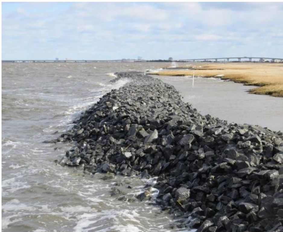
Figure A2-1: Rubble Mound Breakwater Structure at Shooting Island in Ocean City, NJ
