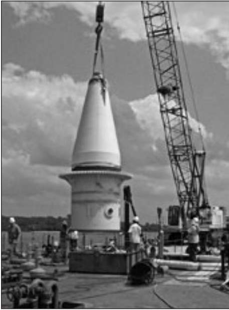
The Marine Design Center teams with workers at the Corps' Ensley Engineer Shipyard in Memphis, Tenn. to set the kingpost on the St. Paul District's Crane Barge Leonard prior to load testing
